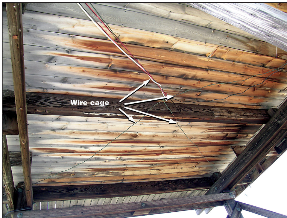
Figure 9—A wire cage provides lightning protection under the floor of a lookout cabin.
