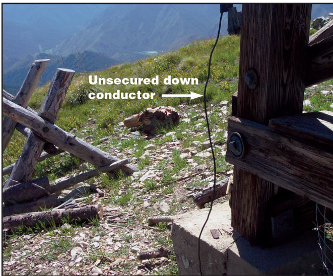
Figure 2—Down conductors should be secured to the structure and not permitted to move or flex.
