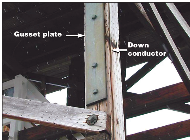
Figure 7—The gusset plate is not bonded to the down conductor.
