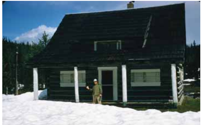
Elk Summit Guard Station third week of June. Our trail crew was first to arrive with the windows still boarded up from the winter elements. Note the two-story cabin with a roof dormer. Trail crews operated out of this station to maintain and reconstruct trails, chase smokes and fight fires, and provide logistical support for Diablo Mountain Lookout and Hidden Peak Lookout.
