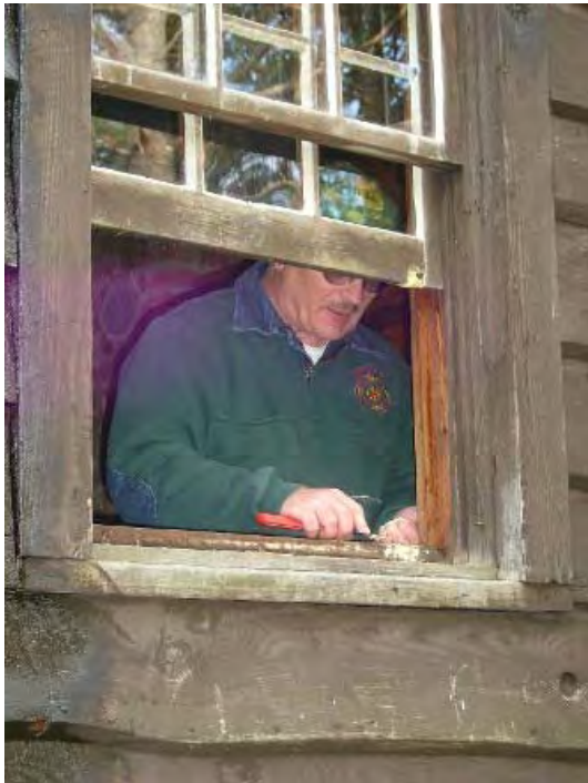
FFLA-NY member and former Page Pond Hill forest fire observer Tom Murphy repairs a window on the cabin.
