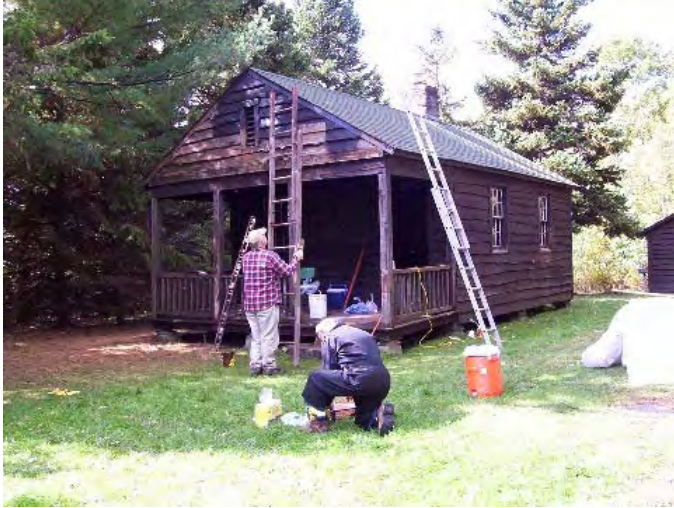
Deputy state director Bob Eckler and Fred Lamb begin staining the cabin exterior.
