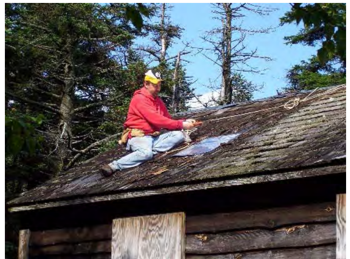
FFLA-NY Scott Eckler temporarily patched the cabin roof.
