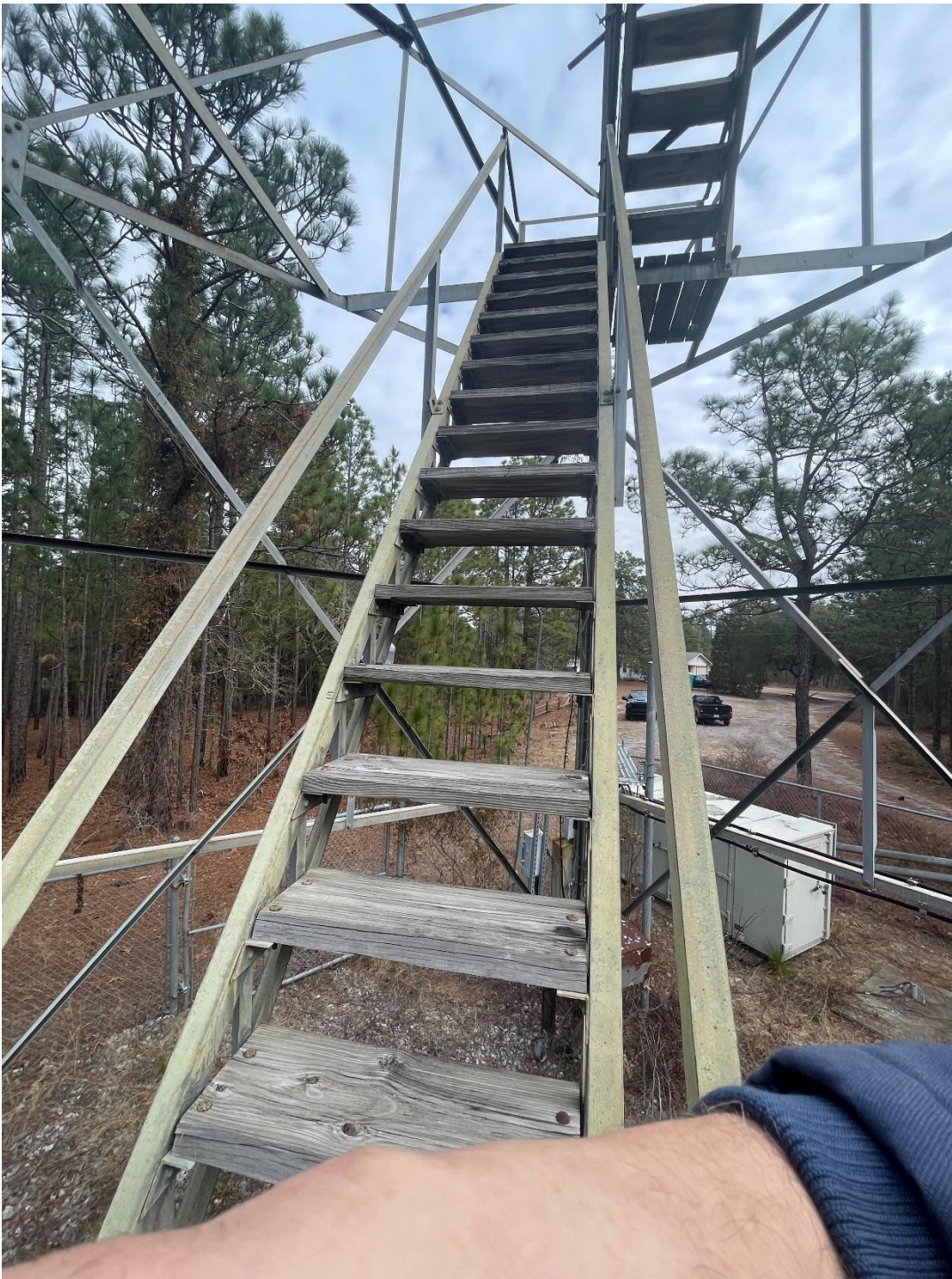
Figure 9. Rosemary Fire Tower, on lower steps, facing east. Note Rosemary House in background.
